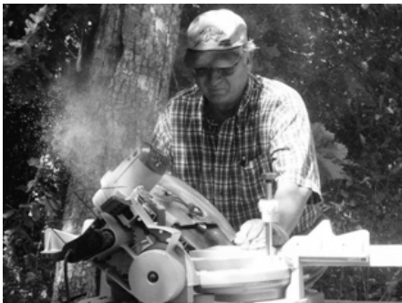
Ron Jenson , new TIA board member, works on the new observation deck.
